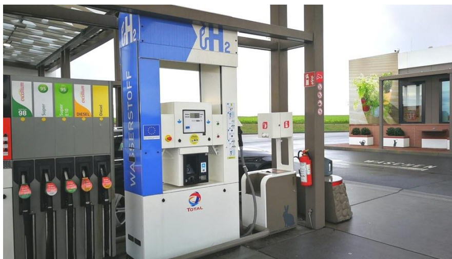
Figure1. Hydrogen filling station in Germany.
